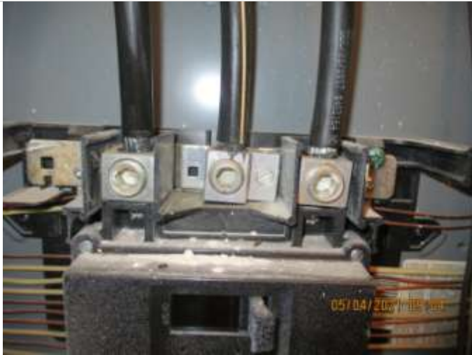
Main Service cables (220v service)
