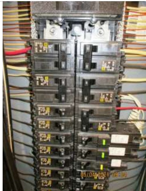
Square D brand panel
