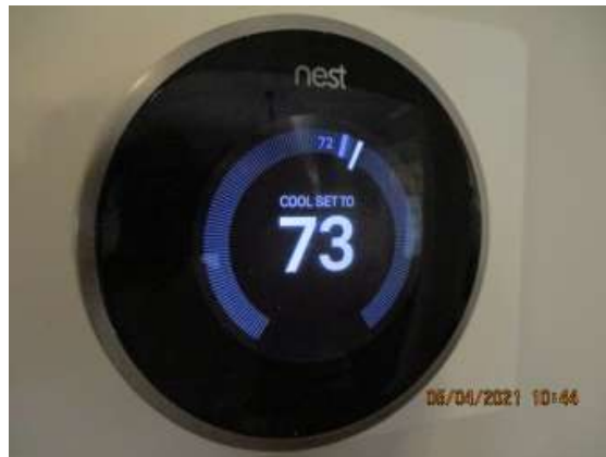
Air system Thermostat – Hallway near Kitchen
