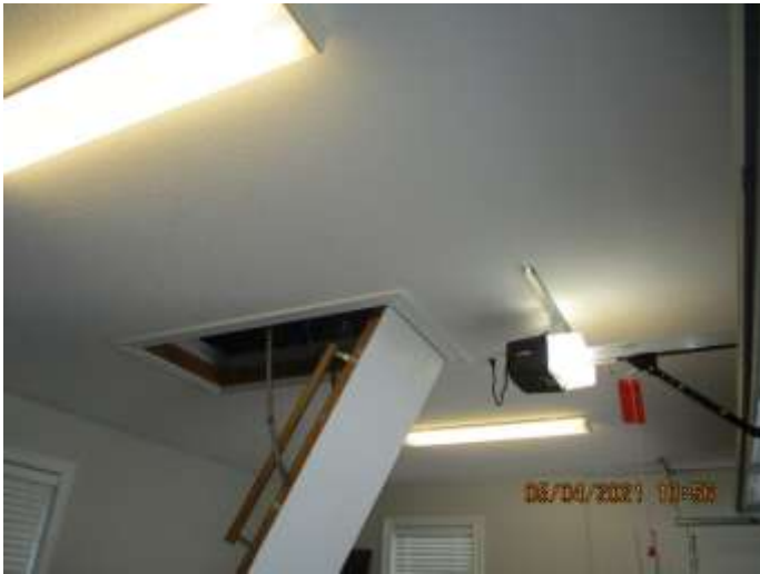
ATTIC ACCESS VIA GARAGE. FYI – Ladder had non-uniform step intervals at bottom.
