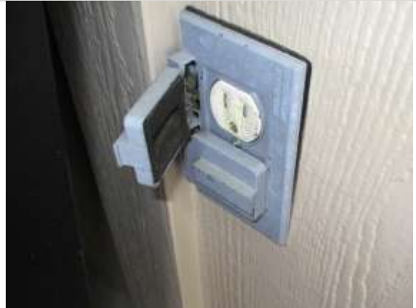
Front door outdoor receptacle is not GFCI. Recommend update receptacle to GFCI + weatherproof.
