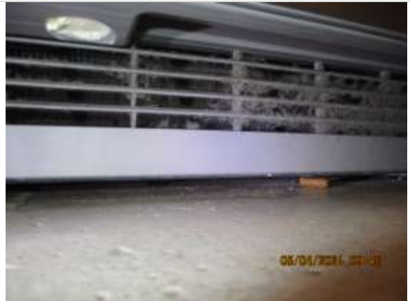
DUST INHIBITS REFRIGERATOR COIL FUNCTIONALITY AND IS A POTENTIAL FIRE HAZARD; CLEAN PERIODICALLY
