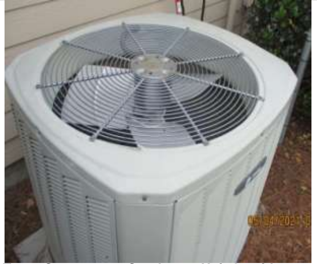
Trane Compressor-Condenser Unit Outside
