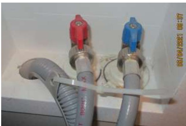
Washer faucets operate normally
