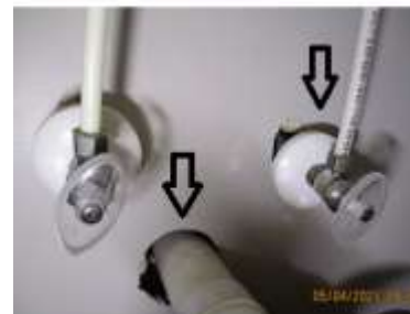
Sealing all plumbing access holes will save energy and stop insects
