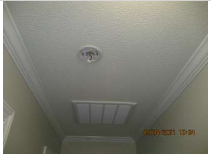
Missing Smoke Detector in East hall
