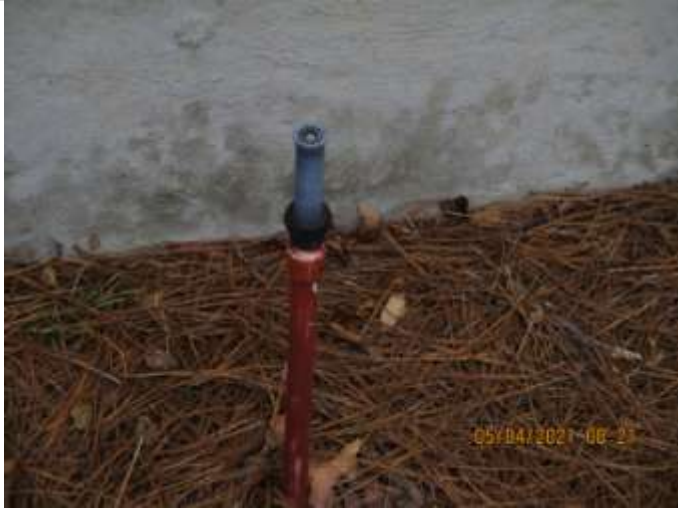
Irrigation system. [ FYI: Ensure no water hits siding! ]
