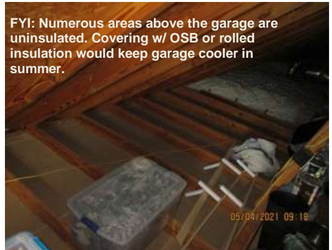
Uninsulated areas exist over garage
