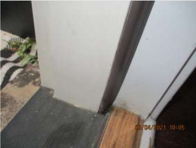
All lower trim boards of door thresholds were solid and free of water damage.
