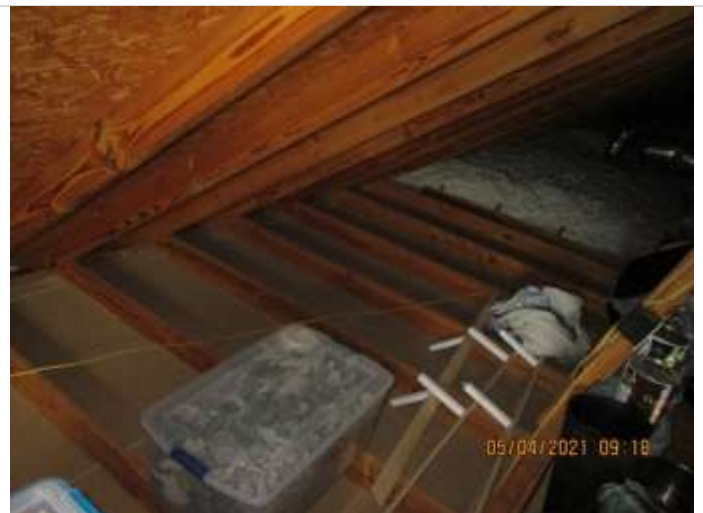
Reminder: Garage Ceiling is not fully insulated. Insulation could keep garage cooler in summer.
