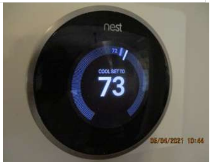
THERMOSTAT - NEAR KITCHEN HALL
