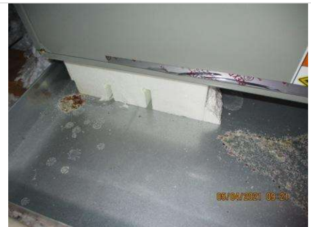
Condensation drip pan is dry. Good!
