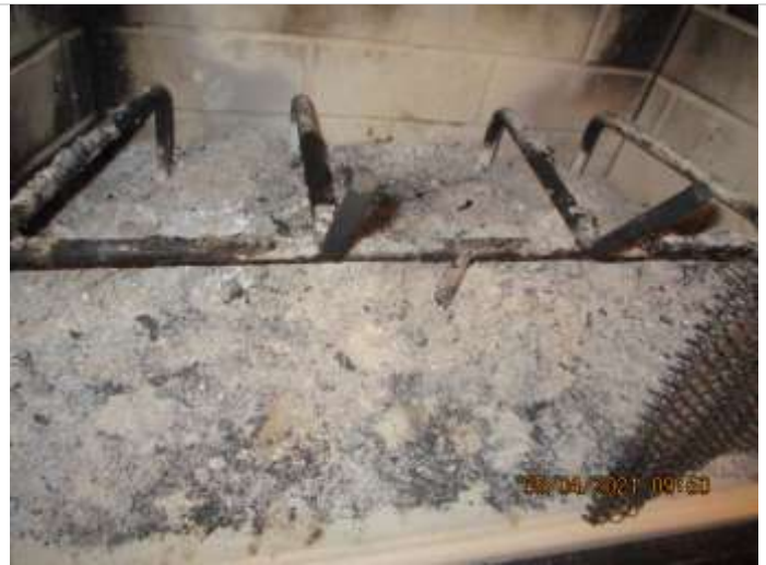
Fire Box floor with ashes
