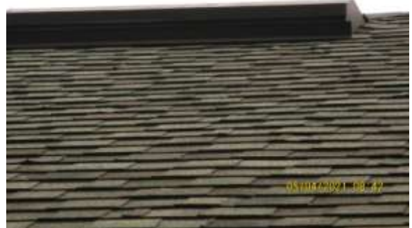
Good shingles are totally flat (like this view), Curling indicates excessive age
