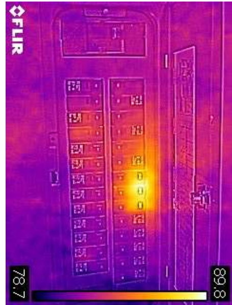
Three AFCI Breakers are Yellow (warm) which is normal
