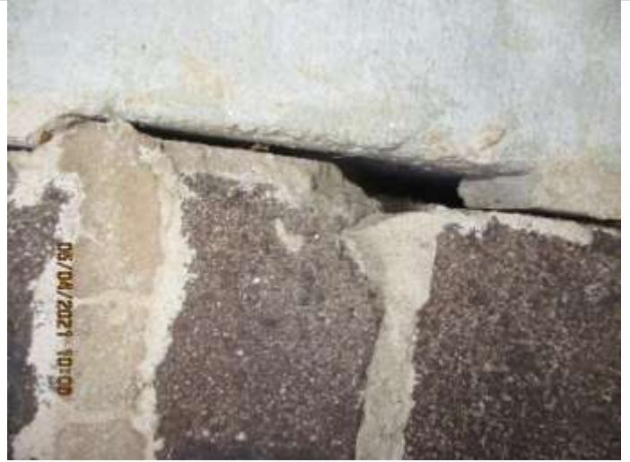
Front steps require re mortar of joints
