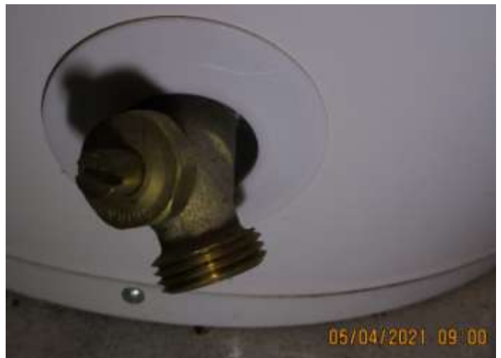
Drain at bottom of tank is missing valve "handle"
