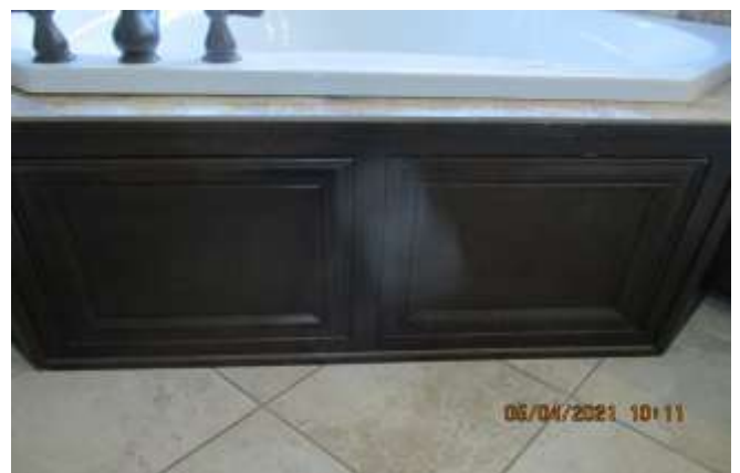
Whirlpool tub should have panel door in front to access water pump (maintenance)
