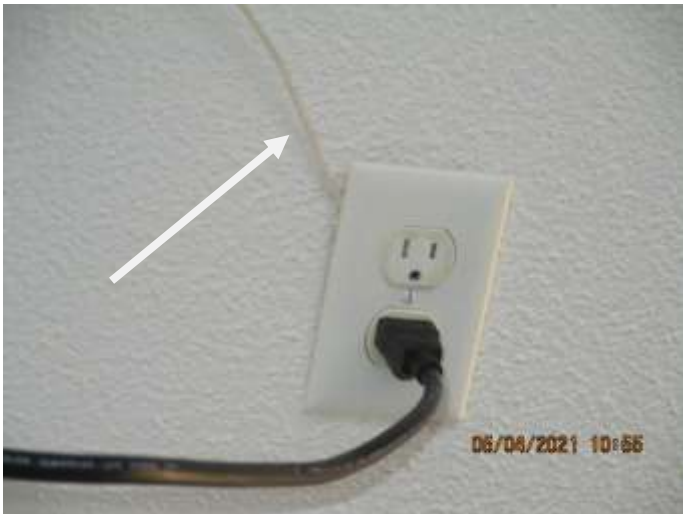
Low voltage wire to wall opener crimped by receptacle plate. Maybe a harmless practice but violates principles of NEC.
