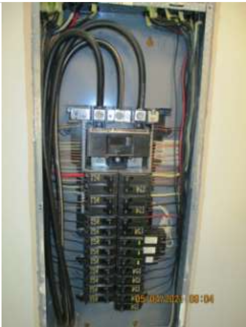
WIRING IS VERY WELL ORGANIZED
