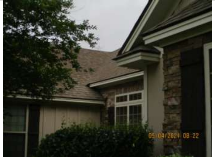
FRONT ROOF - WITHOUT GUTTERS, EXCESSIVE WATER COULD BE AN ISSUE IN FRONT OF HOUSE
