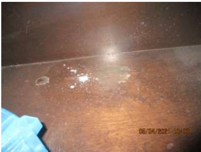
No active leaks under any bath cabinets. The slight water stains here were the only indication of previous drips.
