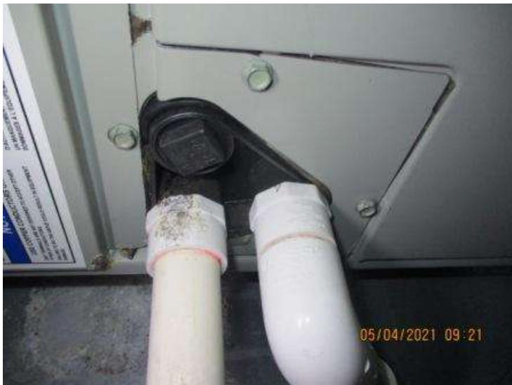
AIR HANDLER CONDENSATION LINES
