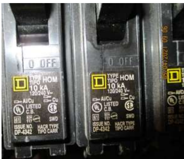
Square D brand panel
