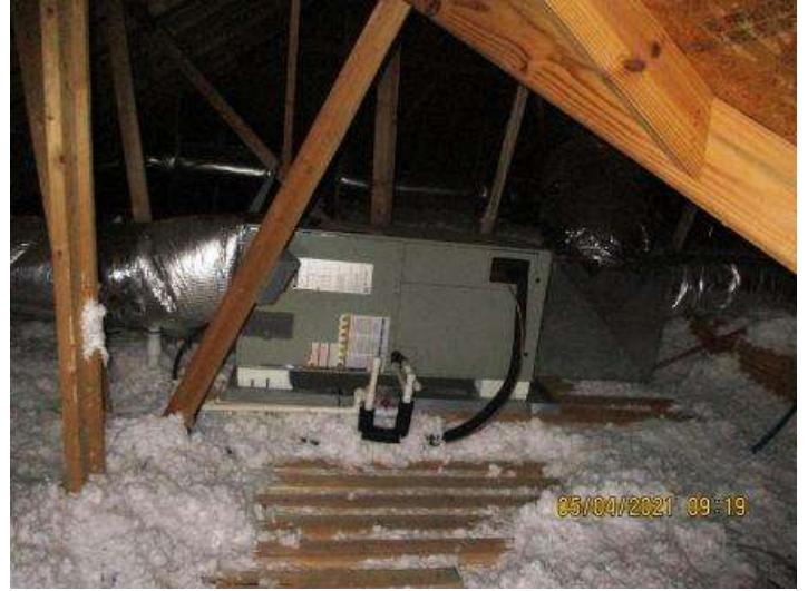
Trane Air Handler (Contains Evaporator Cooling Coils) All AC Components were Functioning
