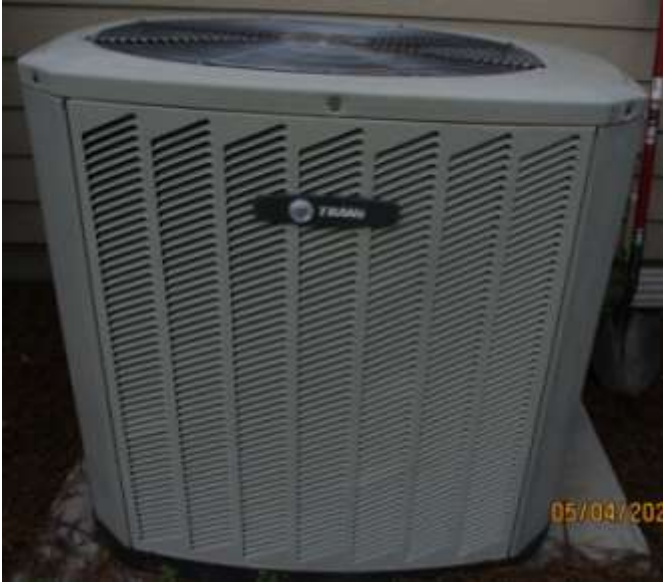
Trane Compressor & Condenser and Compressor
