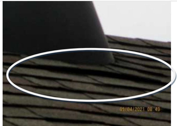
Shingle Buckles Slightly below chimney
