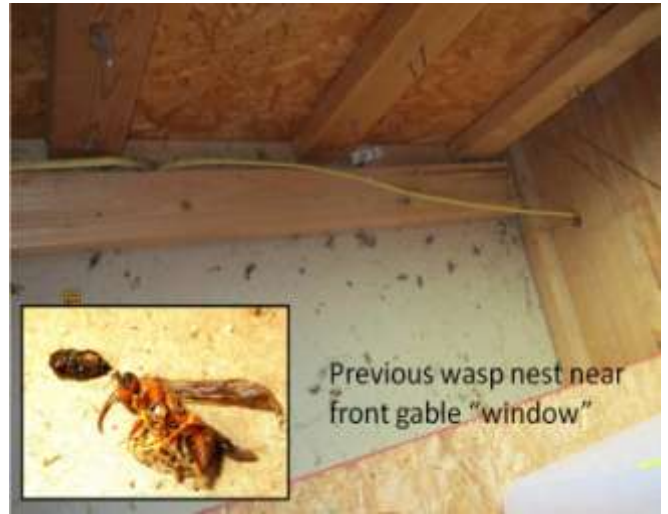
Former wasp nest around front attic window
