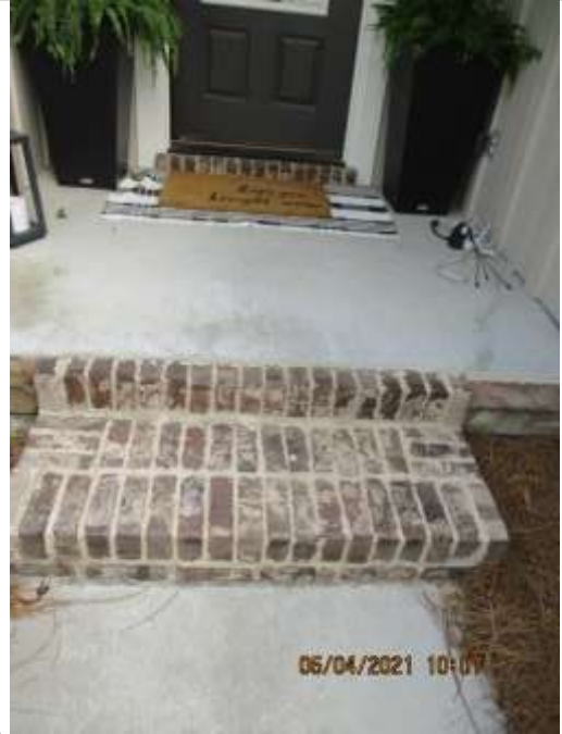
Front steps require re mortar of joints asap.
