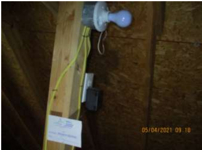
Attic access light & outlet OK
