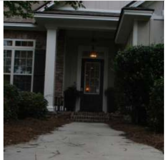
Lacking gutters, the roof valley above entrance is dumping excess water on the brick steps, causing mortar decay.
