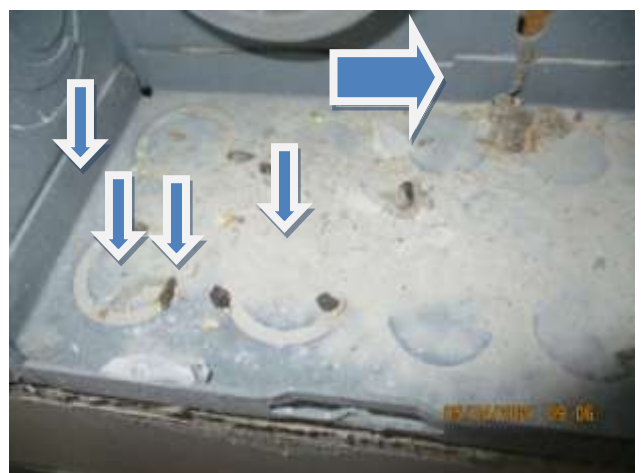
INSECTS CAN BE HAZARDOUS IN ELEC. PANELS RECOMMEND THAT A PROFESSIONAL LICENSED ELECTRICIAN INSPECT & CLEAN.
