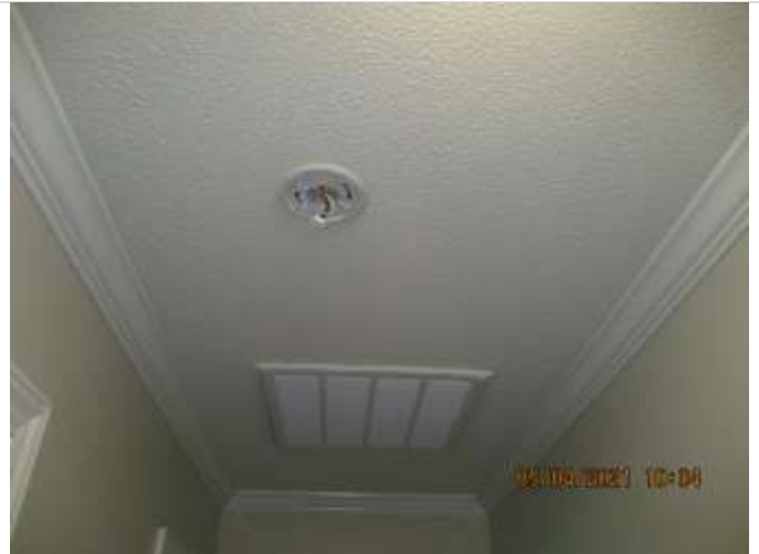
Hallway smoke detector is missing
