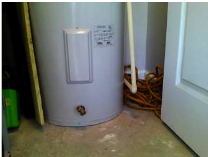
Water heater is missing bottom drip pan.
