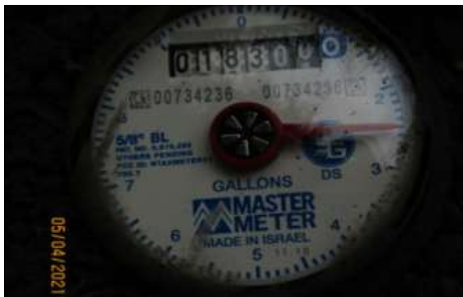
Water Master Meter at Street
