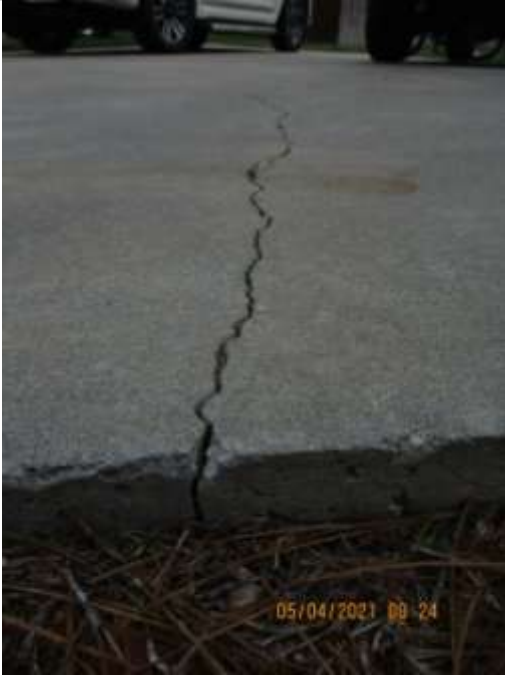
Common driveway crack; can be DIY fill in with appropriate material.
