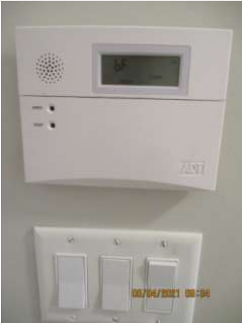
ADT ALARM PANEL AT GARAGE DOOR INSIDE
