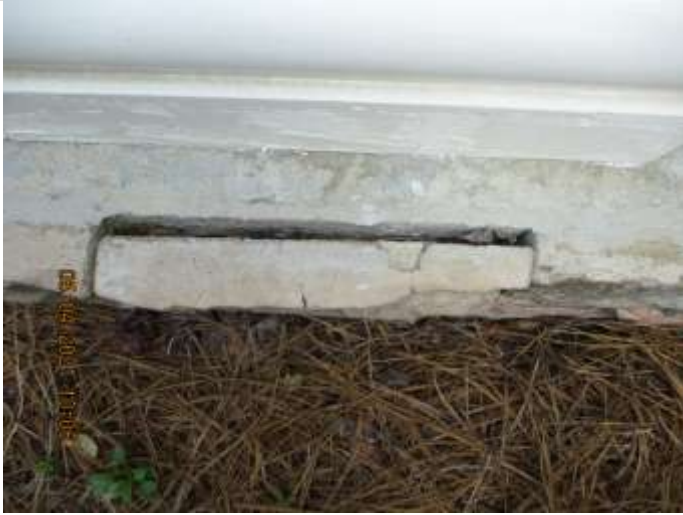
Some décor brick is loose around the front
