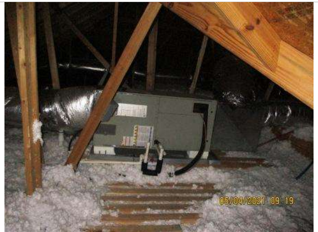
Trane Air Handler in attic. Contains Evaporator Coil that cools air.
