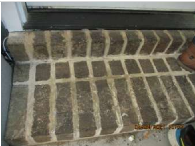
Protected brickwork in garage in very good condition. Compare to front steps.
