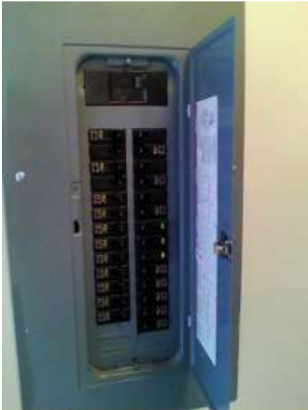
Main Breaker Panel – good condition at front
