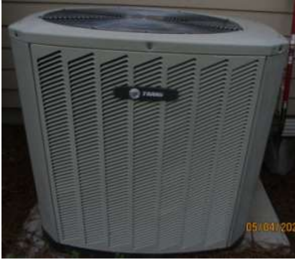
Trane Compressor-Condenser Unit Outside
