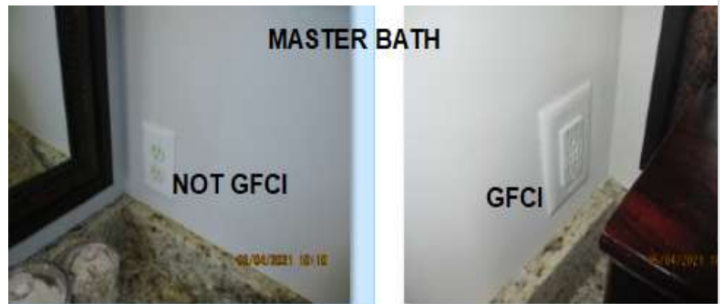
GFCI Receptacle not available on Master Bath counter nearest toilet. Also, missing in Guest bath (below). GFCI can save lives in wet areas.
