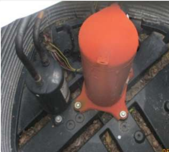
Looking Inside Trane Compressor Unit
