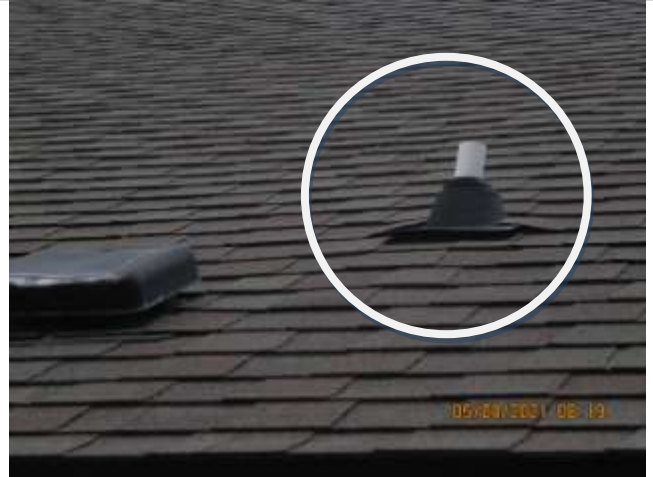
PVC VENT SEEMS TO BUCKLE SLIGHTLY
